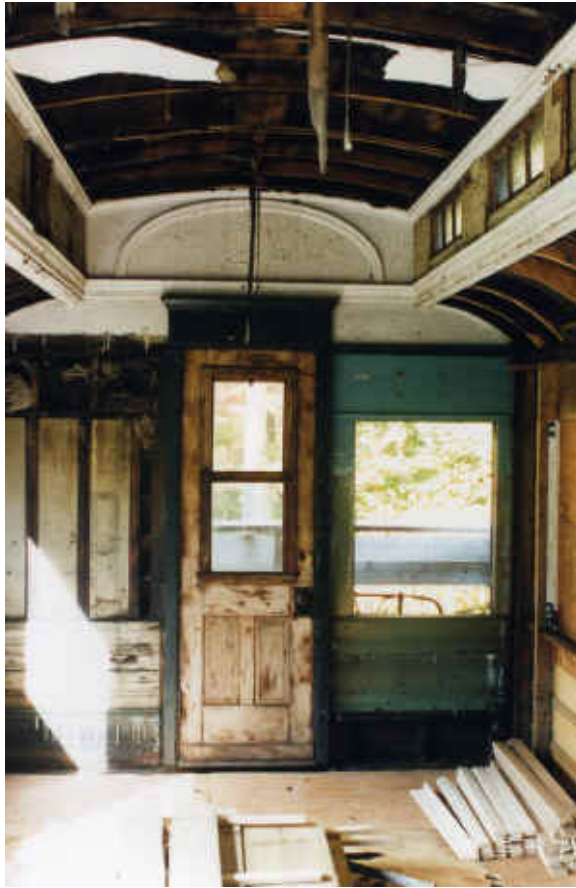
At the start of the project the area where the men's saloon is now looked like this. Note the wasp nests behind the removed paneling near the upper left side of the door.
