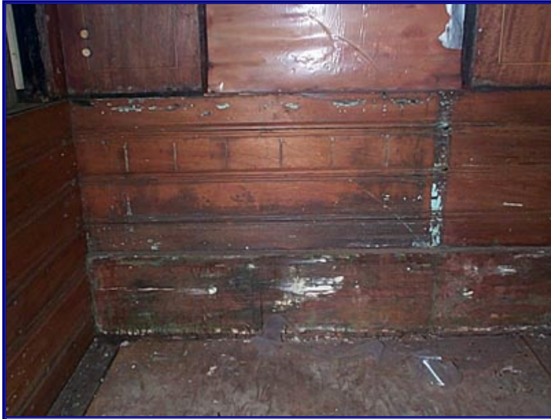
Original wainscoting and base board patched with plaster of Paris, evidently a Steamtown fix. Reasonably effective under paint, but not acceptable with a clear finish.
